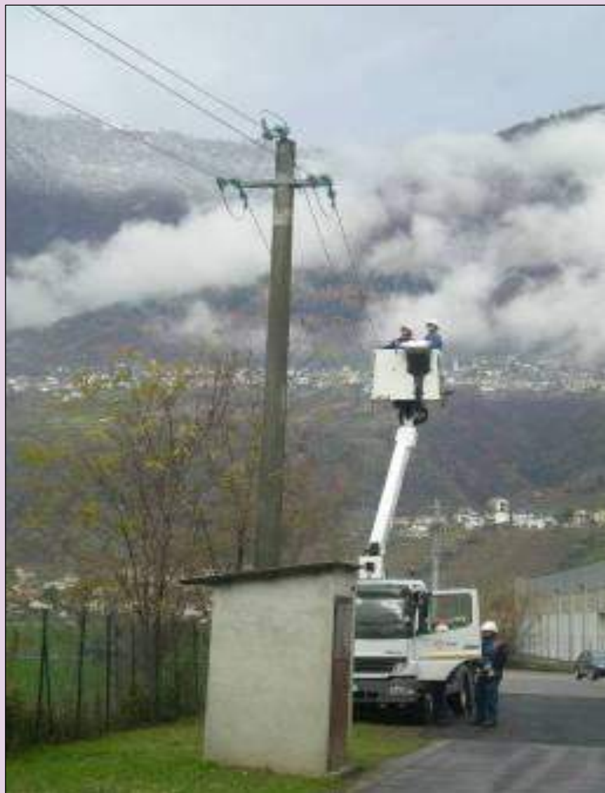
Figure 3. As an alternative to the insulating sheath, the rubber profile EPDM can be applied on MV lines as already done in Valtellina (province of Sondrio). Photo E. Bassi.
